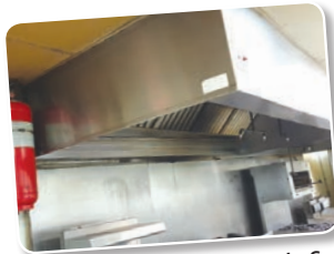
Larkin 20ft hood with fire suppression and blowers
