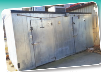
Outside Walkin Refrigerator and Freezer
